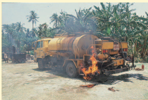
Correct procedures must always be followed when cutting back on site as such operations may be hazardous. Otherwise, fire may be the result. (Bangladesh).
