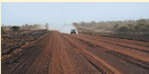
A too excessive aggregate application. (Botswana).
